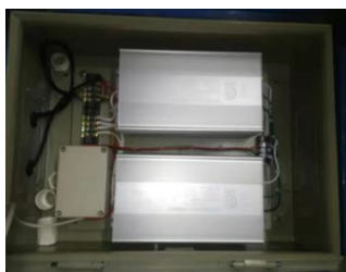
Two Ballasts + Relay
